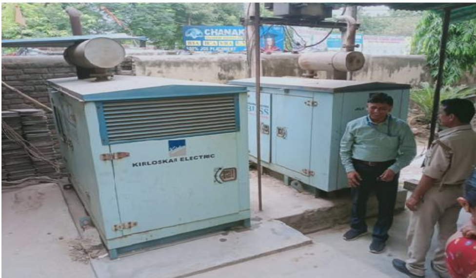
Pic 3: The source of electricity such generators and transformer in old building of the college.
